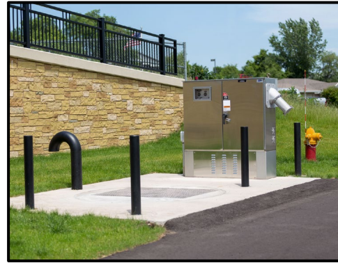
Sewer Lift Station
